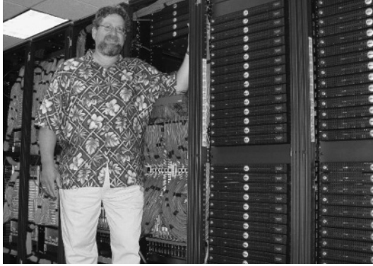
FIGURE 4-27 One of the authors, R. Miller, standing next to several racks of a computational cluster. Notice the racks on the right side of the image consist of a large number of 2U computational units. The three racks on the left and behind R. Miller consist primarily of networking equipment and cables that provide connectivity within the cluster.
