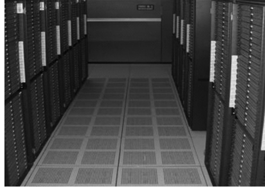
FIGURE 4-28 One aisle showing a number of racks of a very large computational cluster. Notice that the floor consists of perforated tiles, which provide cooling from beneath the raised floor. Note that the nodes in the rack take cooling in from the front and export warm air out of the back. Therefore, in most computer rooms, you will notice alternating cool and hot aisles, where each aisle consists of either fronts (cool aisle; perforated tiles) of two sets of racks, or backs (warm aisle; no perforated tiles) of two sets of racks.
